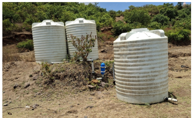
Water Storage Tanks
