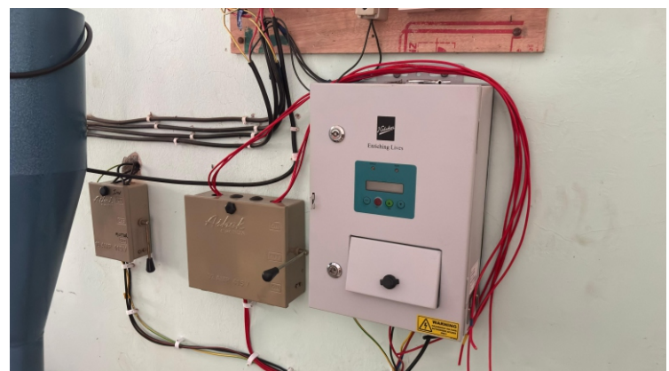
Installed Solar Powered
