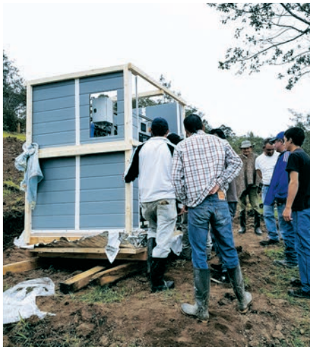
All Partners Carried Out Installation and Connexion of Filtering Unit
