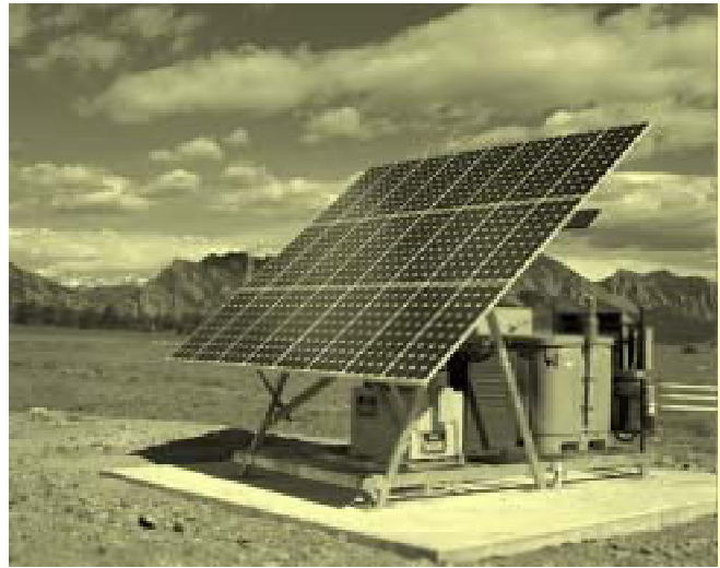
Several technologies can often be used together in a RAPS system, such as this PV-diesel hybrid.
