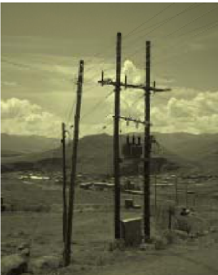
Small renewable energy systems can often be a better option than extending centralised electricity grids.
