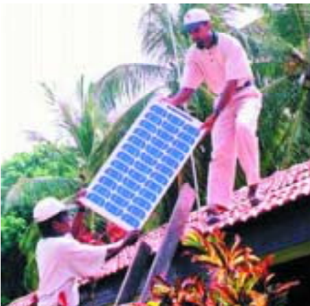
A one module solar home system is installed in Sri Lanka (courtesy SELCO)
