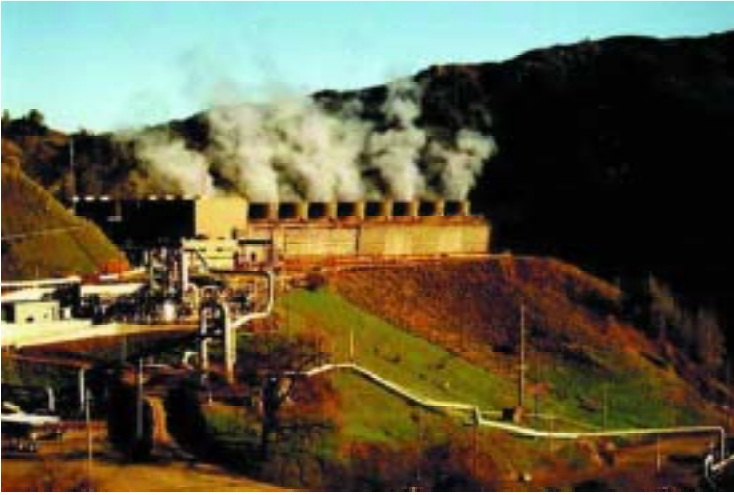
A geothermal energy field. (Courtesy NREL)
